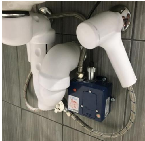
Figure 8. The underneath of a sink in a Texas A&M University – Corpus Christi restroom.
