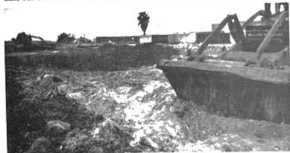
Demolition of old structures signals the beginning of campus expansion for four-year status in 1994. Photo by Javier Fonseca.
