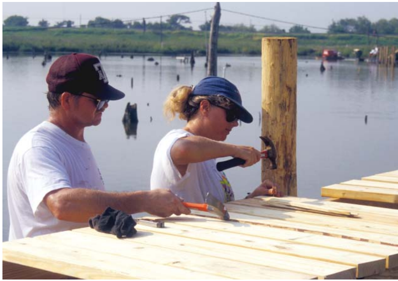
Figure 9. Dr. Roy Lehman and Terri Nicolau building walkways in Parkers Cove, San Jacinto, Texas.
